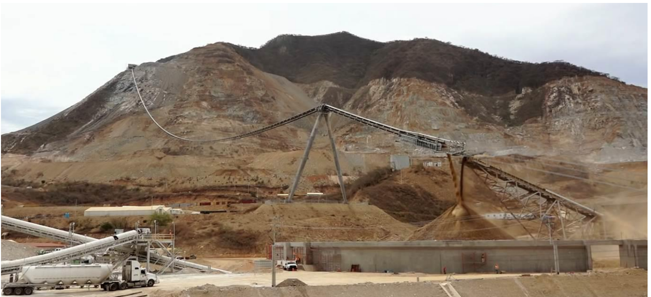
View of a RopeCon installation pictured at El Limon-Guajes, Mexico demonstrates the systems minimal footprint in difficult terrain.
