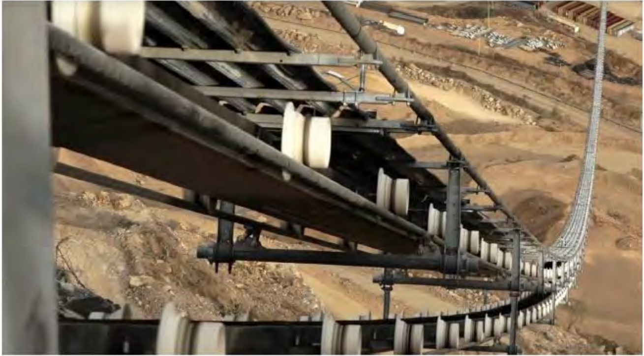
Figure 30 Close-up view - RopeCon transports material on a flat belt with corrugated side walls that is fixed to axles that run on track ropes suspended from tower structures.
