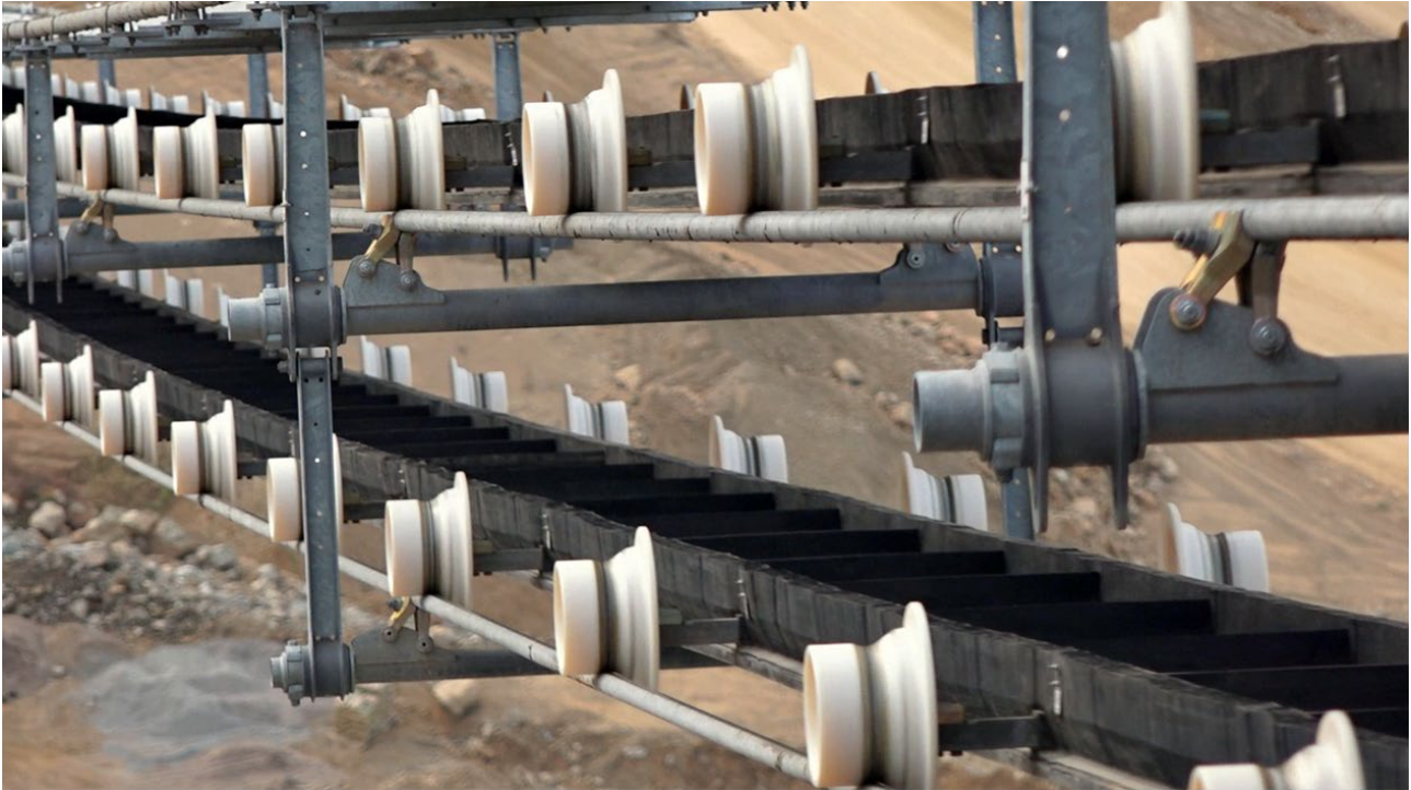
Figure 18.4 : Close-up view - RopeCon transports material on a flat belt with corrugated side walls that is fixed to axles that run on track ropes suspended from tower structures.
