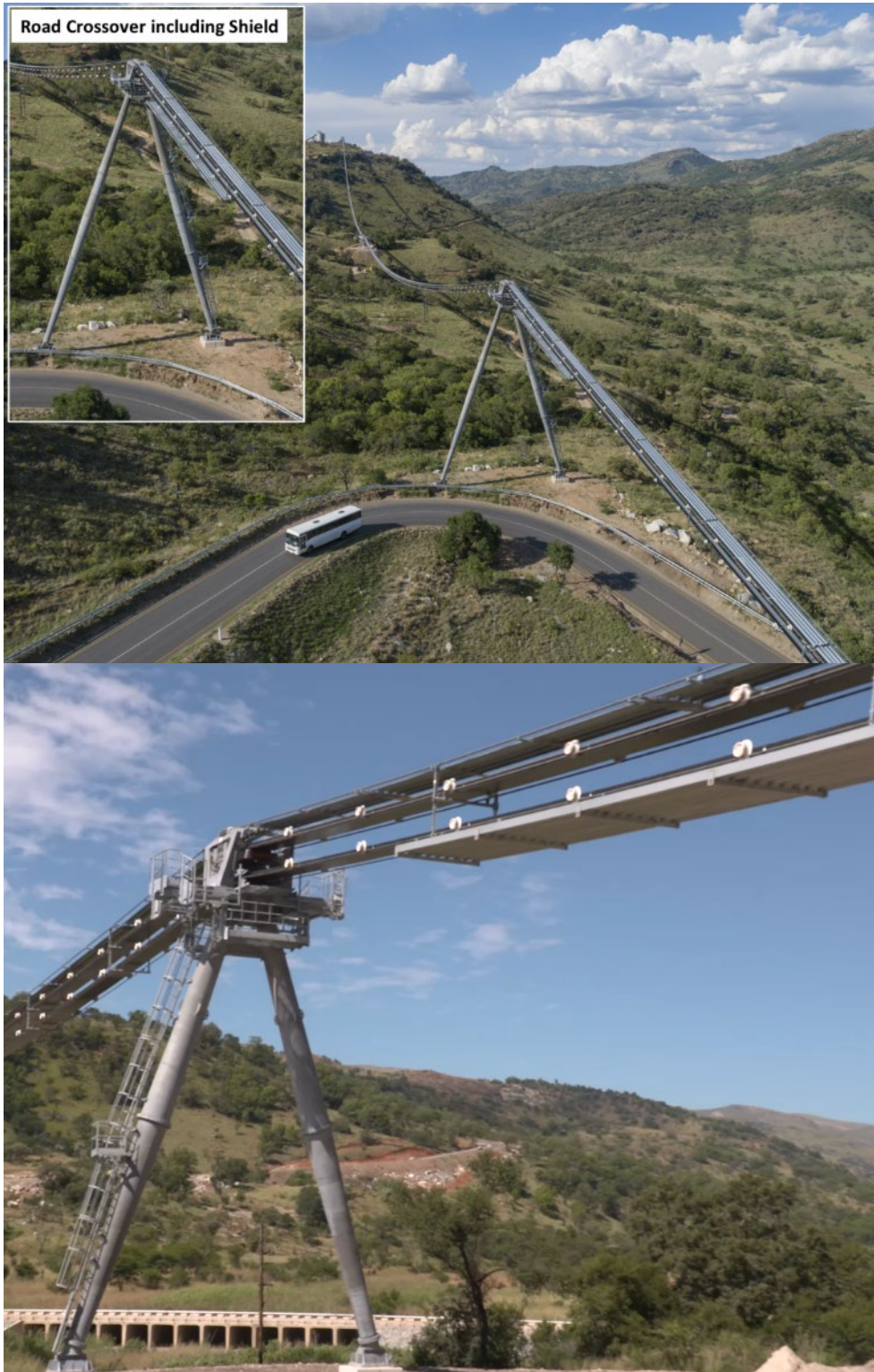
Figure 18.5 : View of RopeCon Road Crossing Installation Pictured at Booyensdal North, including Close-up of Shielding (below conveyor) for Road Protection.
